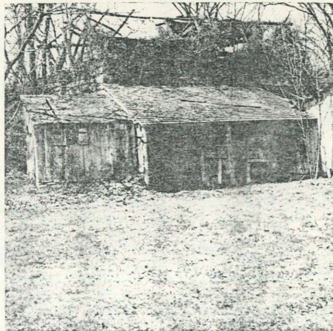
Limekiln showing adjacent sheds and roof structure built over opening below where lime is removed and remains of roof above which protected shaft openings. Located on farm near Harpers, Lebanon County.
