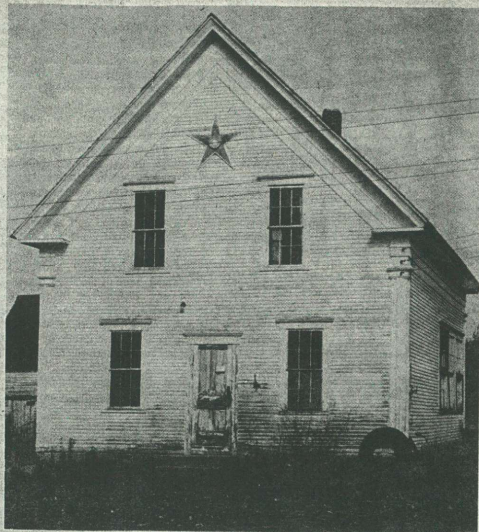
MEETING HOUSE in Stannard is an old school building which demonstrates the rigors of the years with its faded paint and need of repair.
