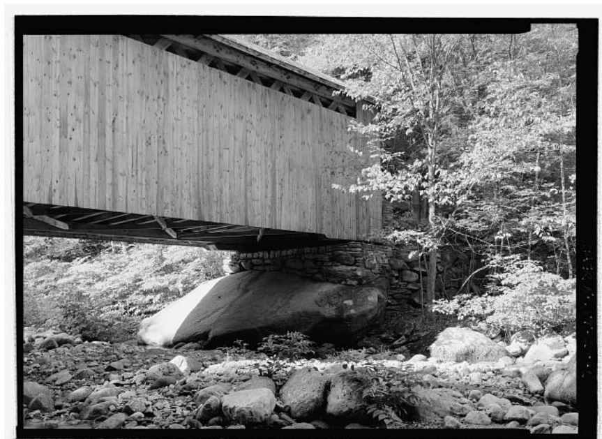
BROWN BRIDGE. Southwest abutment detail from downstream. Photograph by Jet Lowe, 2004 [HAER VT-28-6]
