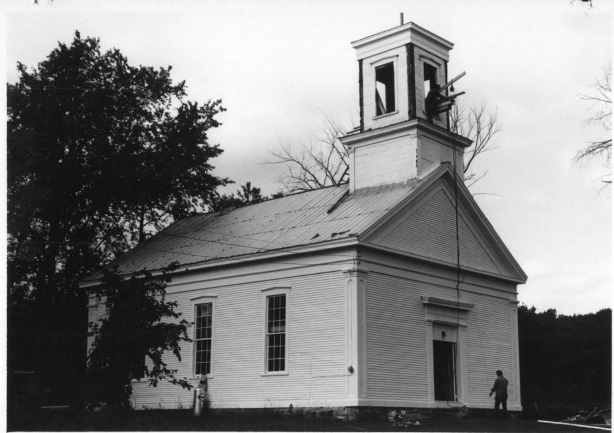
Historic view, July 1977, looking southwest at the front (north) and side (east) elevations of the East Monkton Church. Note the work being done on the tower. This is presumably when the gable roof on the tower was changed to a pyramidal roof.
